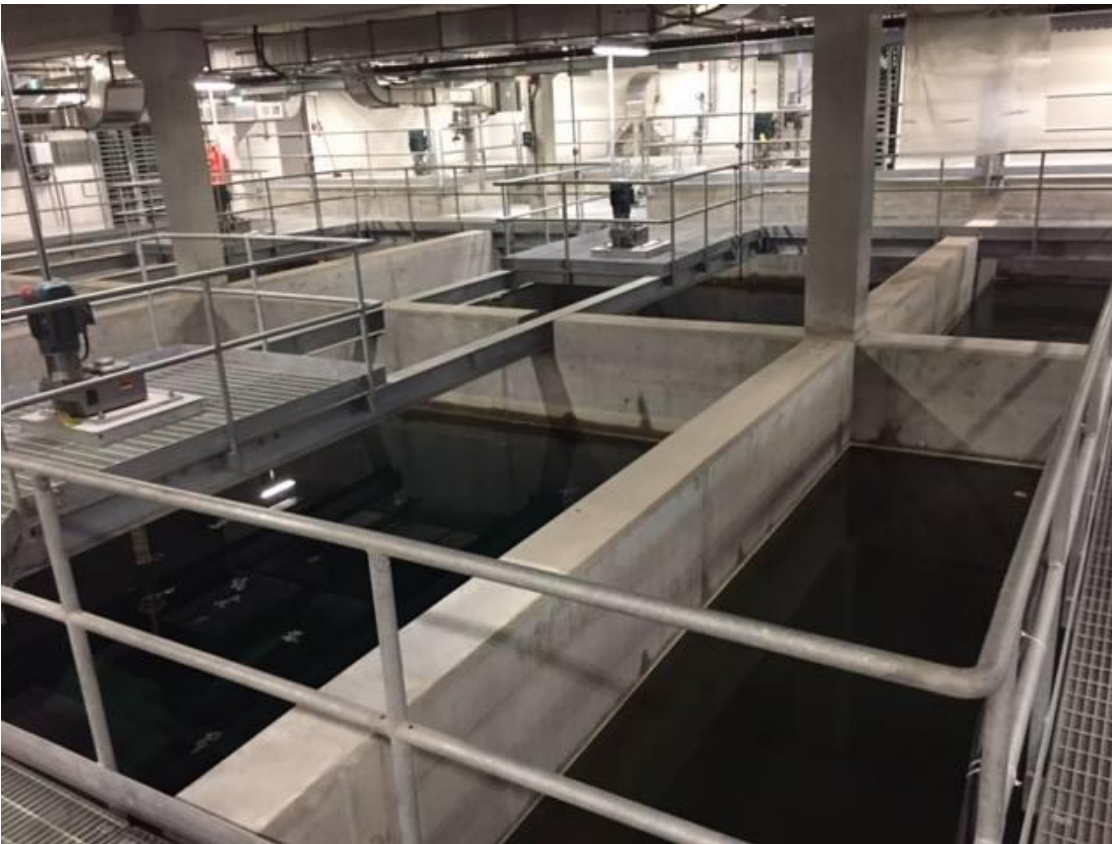
Figure 6: Mixing and Flocculating Tanks Prior to Solids Removal in Dissolved Air Flotation
