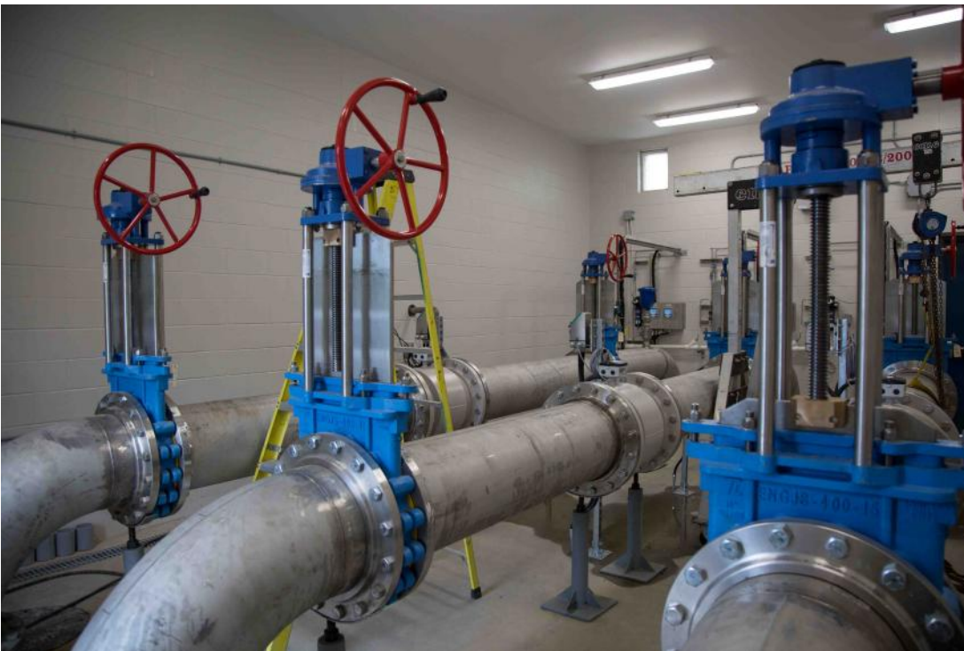
Figure 2: Interior of the New Groundwater Supply Pumphouse
