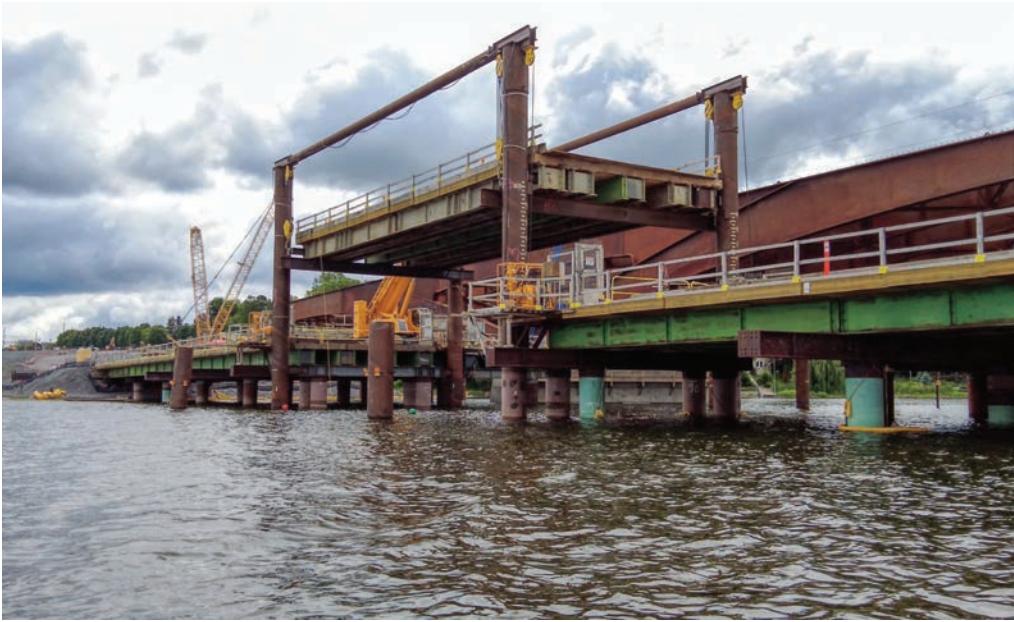
The project team's hybrid approach included a temporary lift-bridge over the Cataraqui River.
