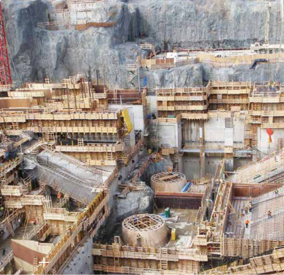
Smoky Falls: Scale of the site before pouring the concrete. View of circular formwork for Units 1 and 2, the only formworks that were so complex they had to be made in a factory.
