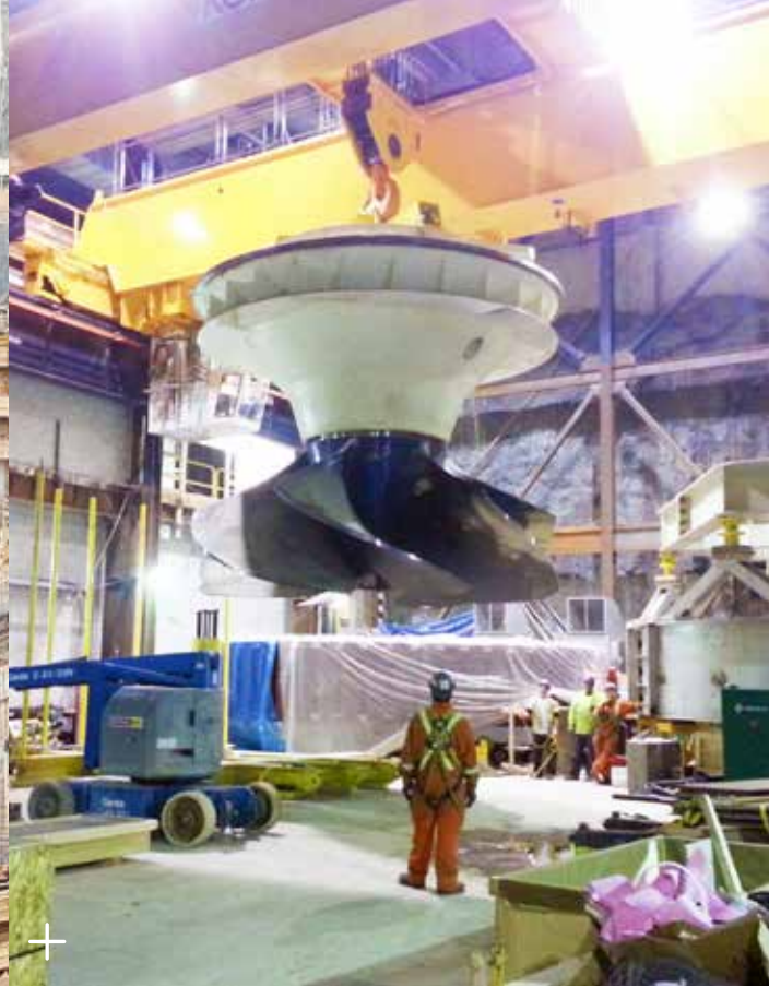
Smoky Falls: Installation of a turbine with the help of the 275-ton bridge crane.
