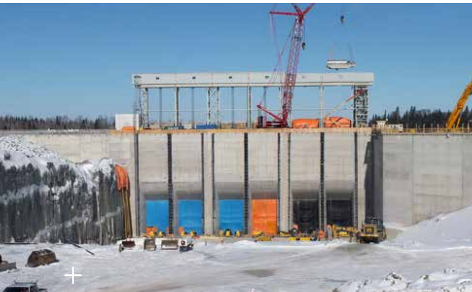
Smoky Falls: Upstream view of the six intakes serving the three units of the new station (March 2014).
