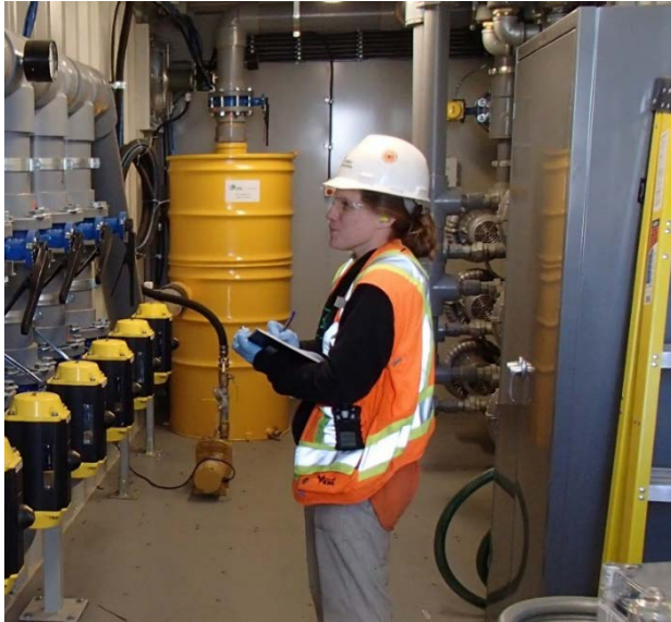
Photo 3: Air extraction system
