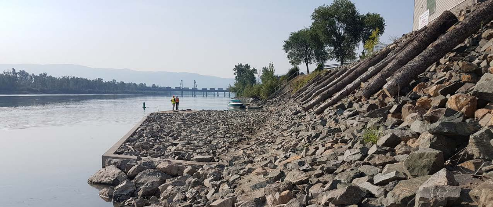
Riverbank armoring and wedge style intake to control erosion
