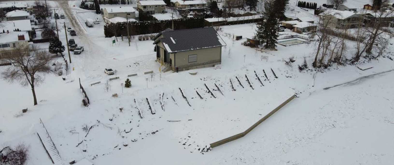
Very low river flows in winter, exposing the intake structure to flowing ice
