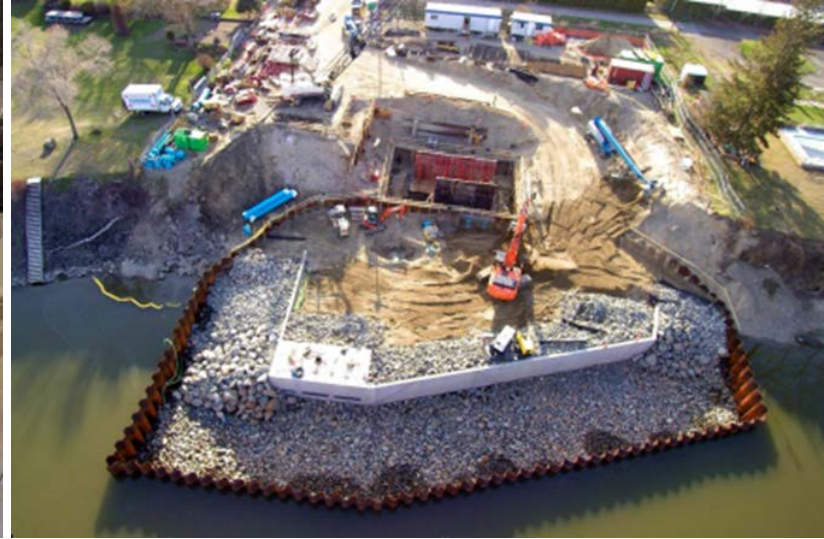
Deep construction below the water table required intensive attention to constructability and the sensitive river habitat
