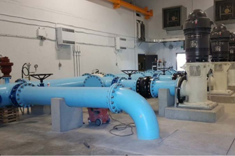
Pumphouse interior showing 300 kW vertical turbine pumps
