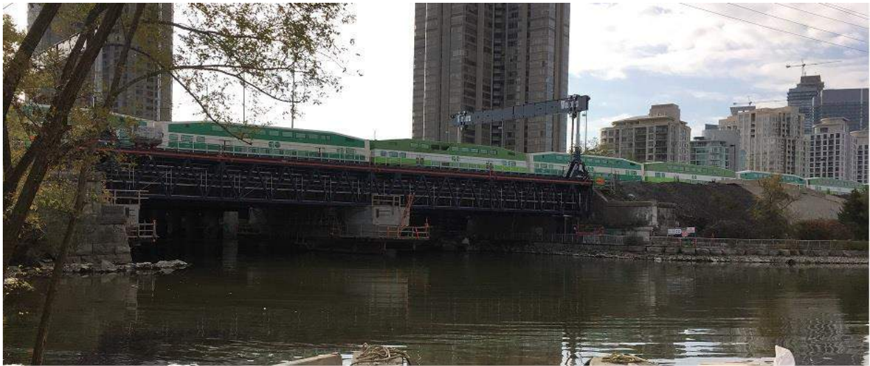
Figure 5: Humber River Bridge open for revenue service following a weekend work block.
