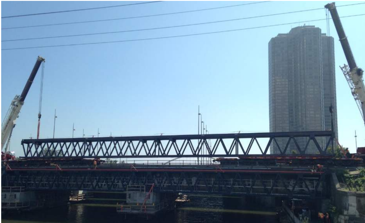
Figure 1: Cranes lifting half of the gantry truss system in to place on concrete corbels.
