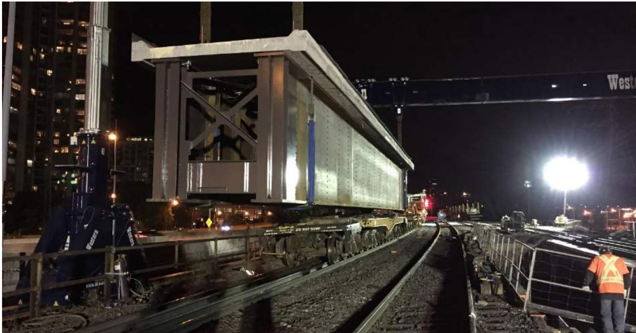
Figure 4: A new span being lifted into position during of the 50-hour weekend closures.
