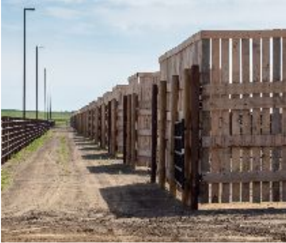
Pen alleys, gating, and lighting designed for optimal handling conditions and safety
