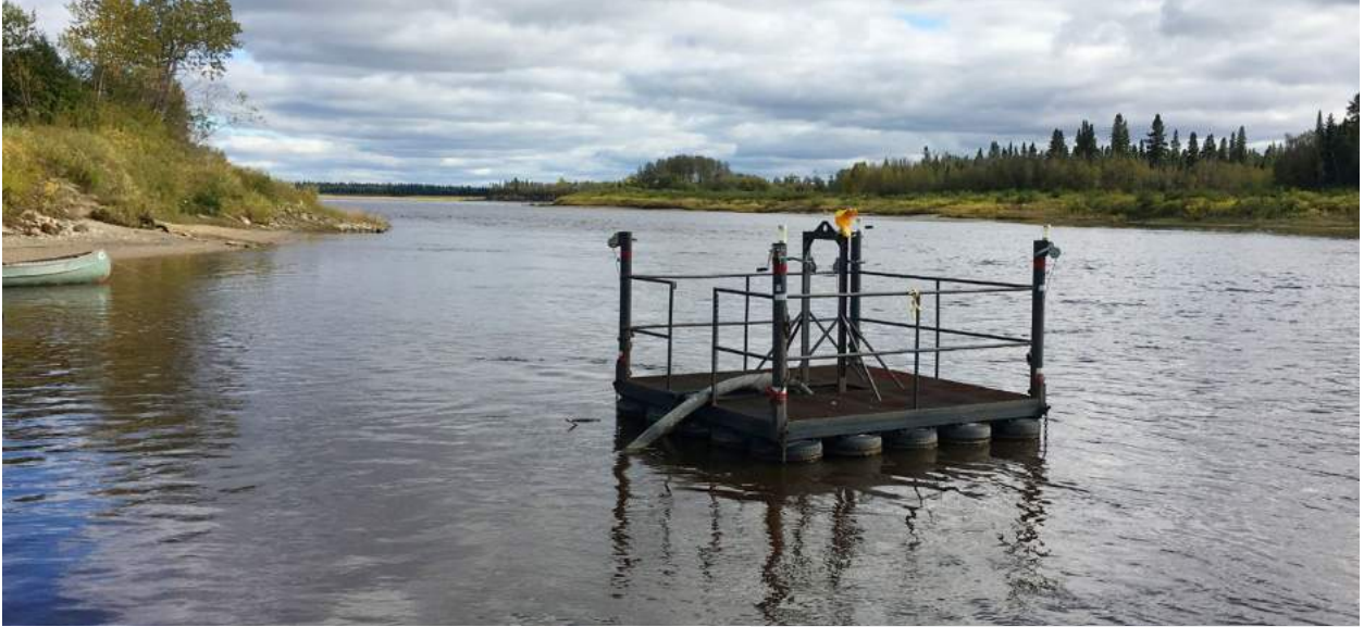
Temporary raw water intake for the Moose Factory water treatment plant.
