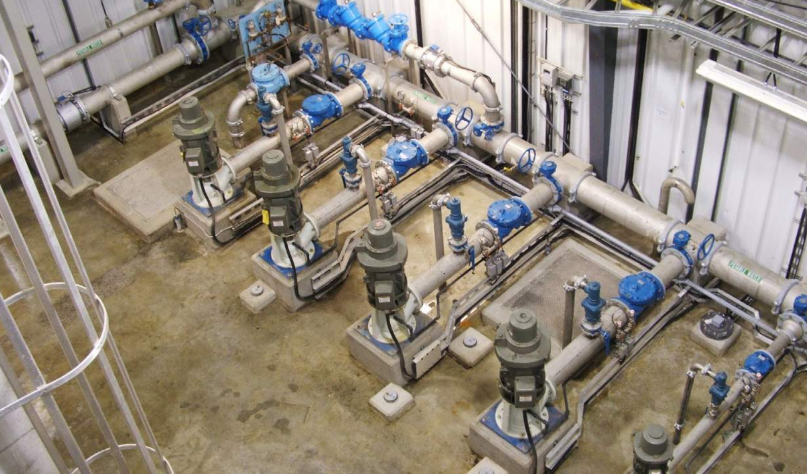
Treated water pumps, Oneida Nation of the Thames water treatment plant.
