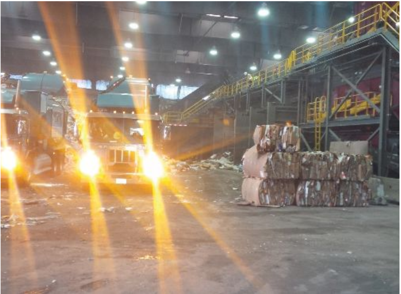
Waste reception and sorting hall
