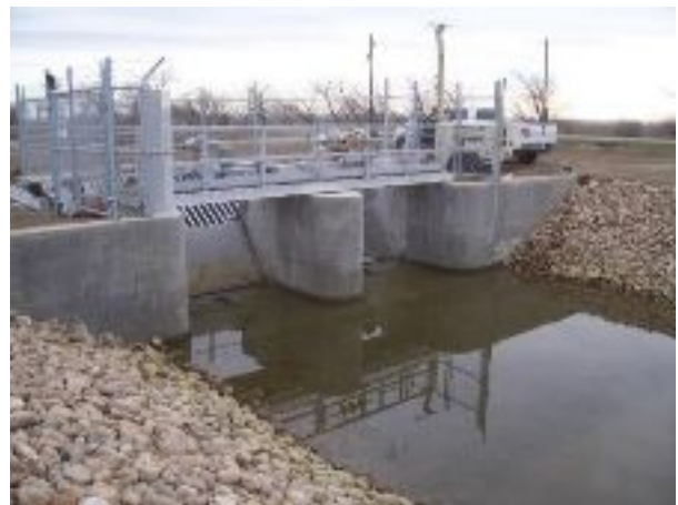
Inlet Structure with Automated Overshoot Gates
