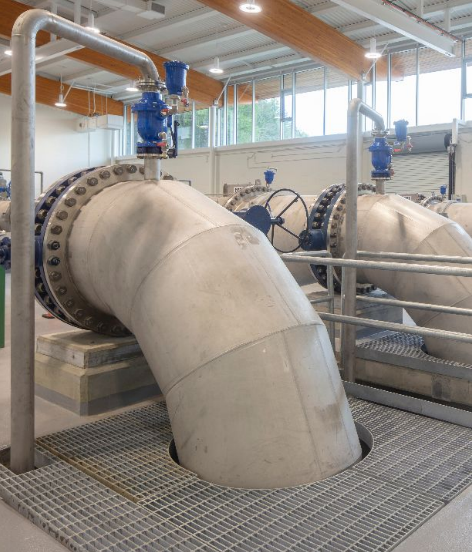
UV disinfection system
