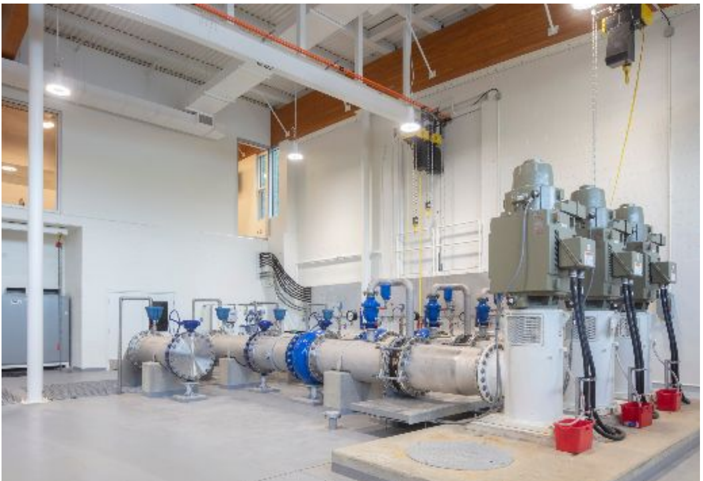
Vertical turbine pumps
