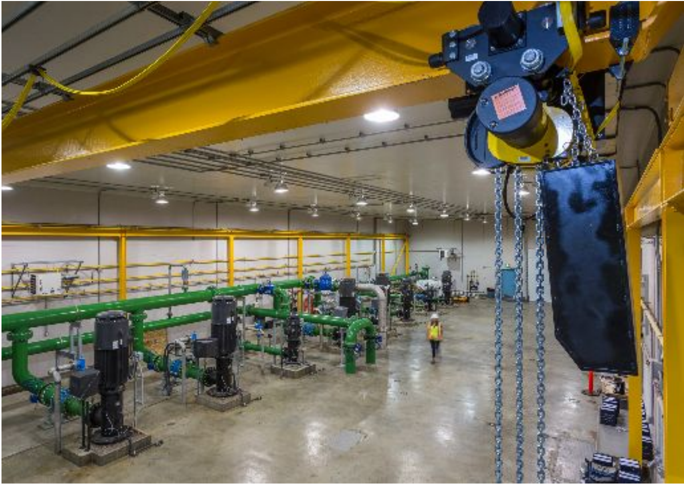
Zelma Pump Station
