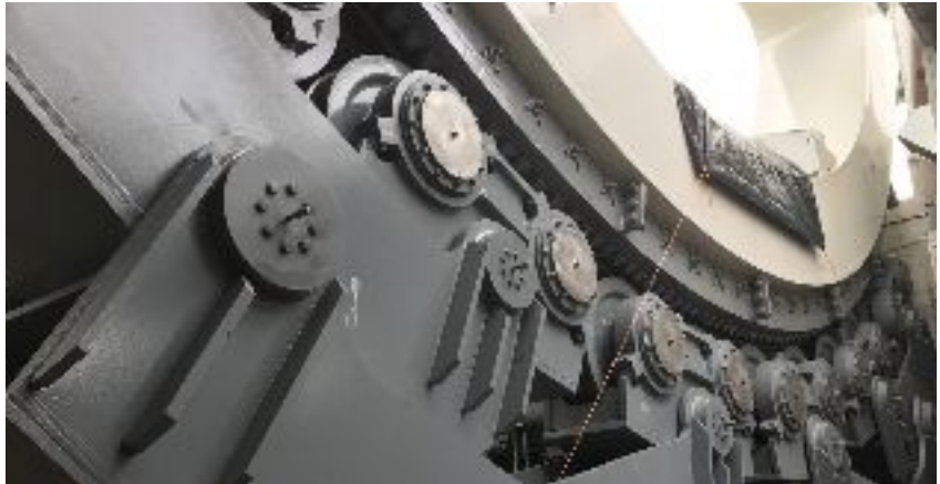
Close-up of the Span Support Roller Assembly and Rack Support System
