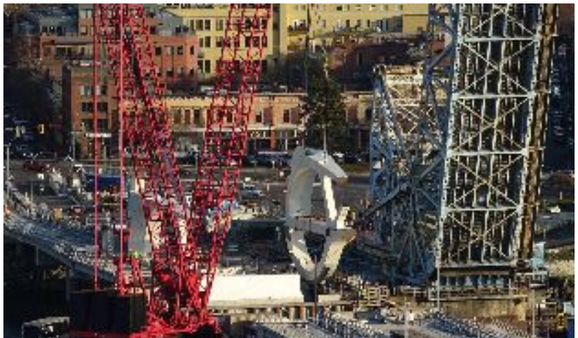
South Ring of the Moveable Span being set in place by the Dynamic Beast - a 900 tonne floating crane
