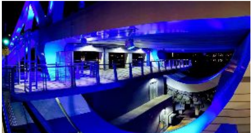
Nighttime view inside the bascule pit showing the span support roller assembly, rack support gear teeth and pedestrian walkway through the rings.
