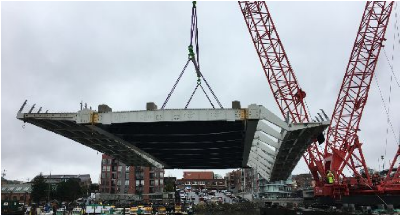
Orthotropic Steel Deck with Pedestrian Walkway and Multi-use Deck attached being lifted into position by the Dynamic Beast - a 900 tonne floating crane
