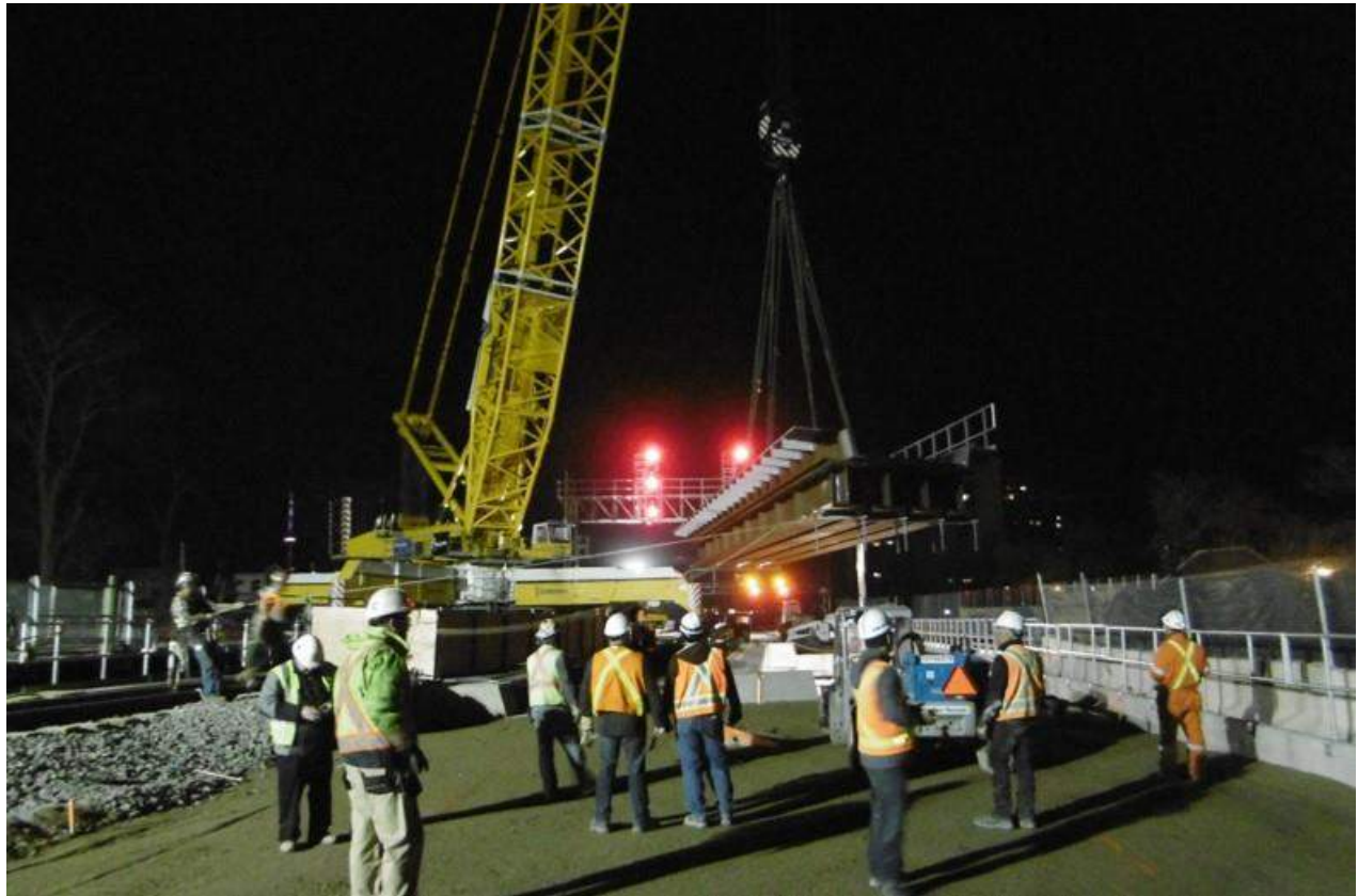
Figure 1: New span being lifted into place by crane during a weekend closure.
