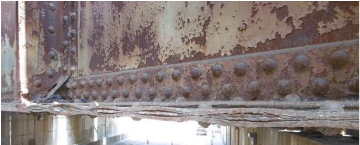
Figure 4: Deterioration of the existing structure. This material was recycled following its removal.
