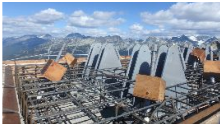
>> Rock Anchors and embedded cable anchor plates for the Skybridge west abutment slab.
