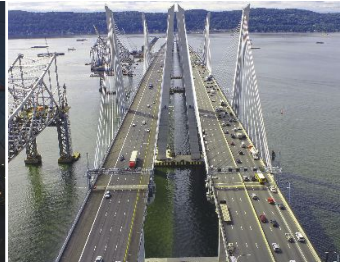
The iconic V-shaped towers, complete with architectural chamfered tops, will provide efficient A-frame action to support the future installation of a cable-stayed commuter rail bridge between the twin structures.
