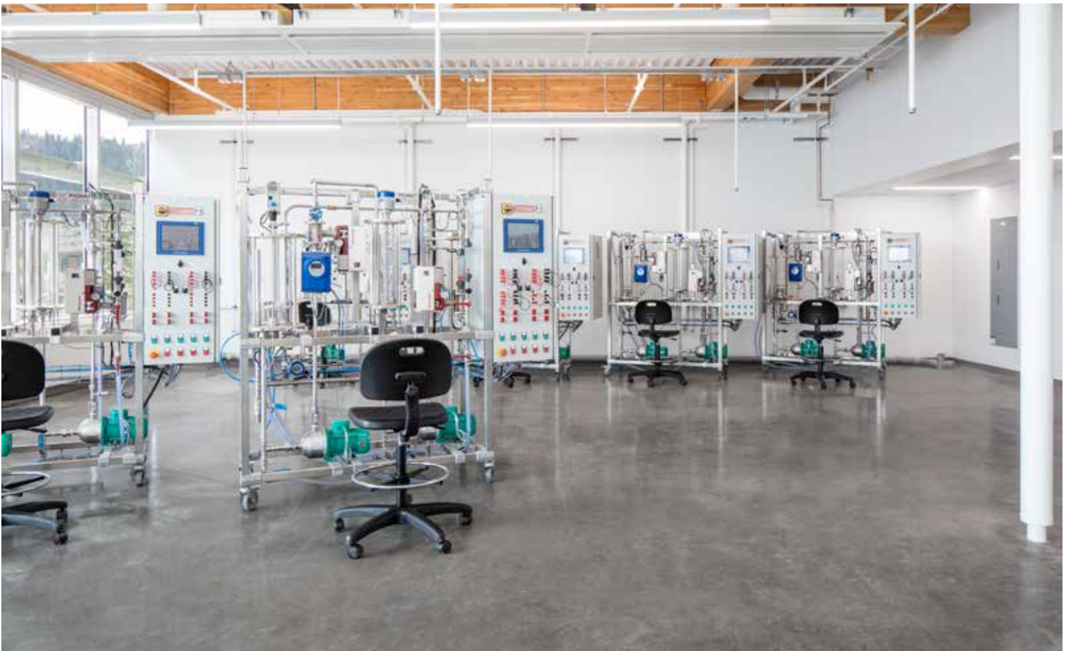
Instrumentation Lab with Active Chilled Beams
