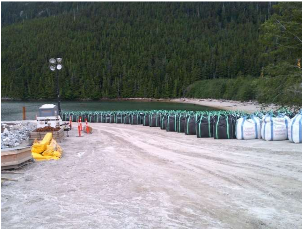
Image 12: Cement bulk bags off-loaded and awaiting transport to cement slurry mixing station
