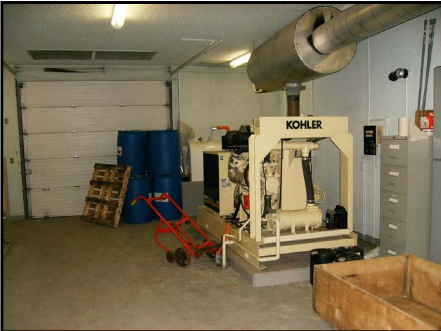
4. Original Genset Location
