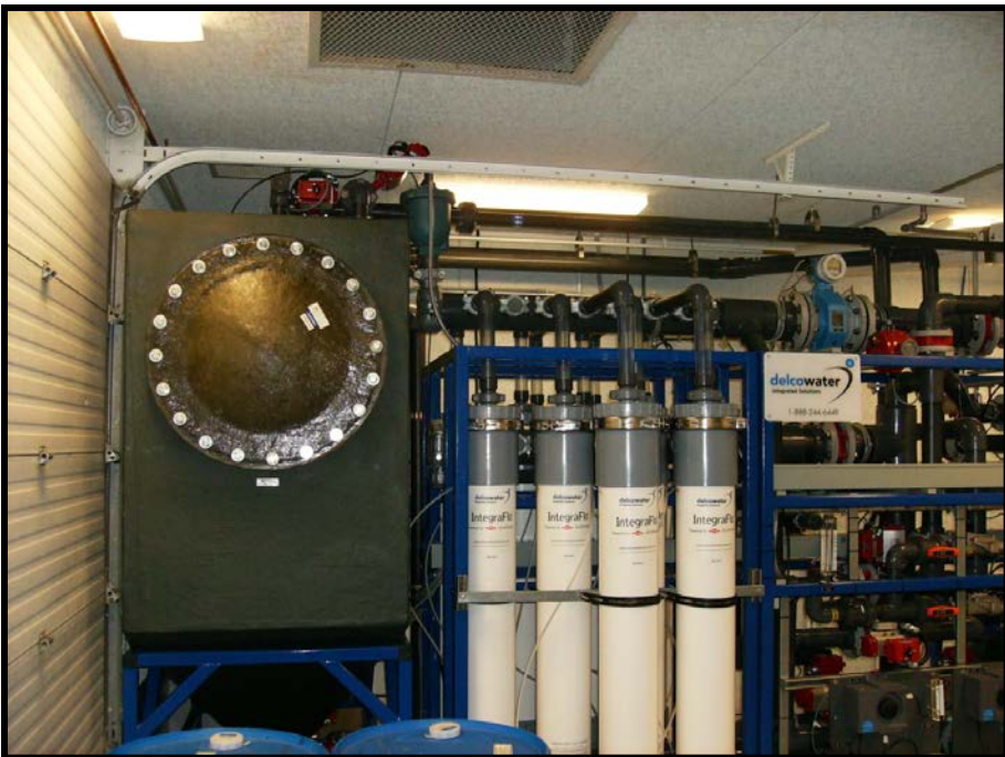
6. Ultrafiltration Membrane Treatment Unit
