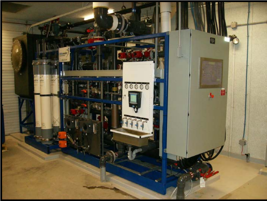
5. Ultrafiltration Membrane Treatment Unit
