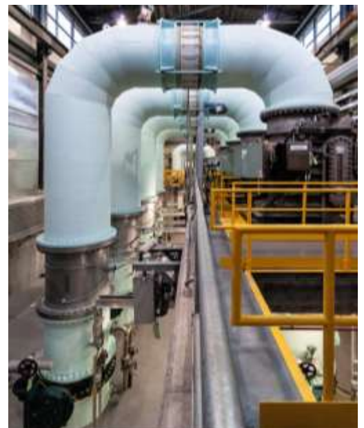
Vertical pipe loops
