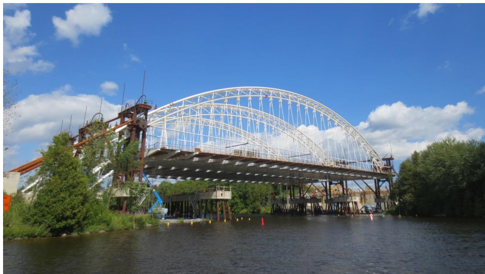
Figure 8. Launched bridge structure supported on lift towers prior to lowering onto thrust blocks.
