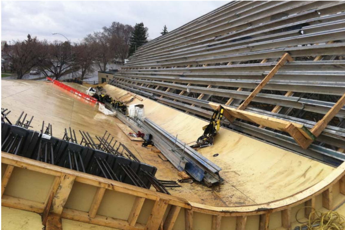
Figure 3: Construction of post-tensioned troughs, which allowed for an undulating free-form concrete roof. Note Isokorb material at edge of roof. Credit: Hughes Condon Marler
