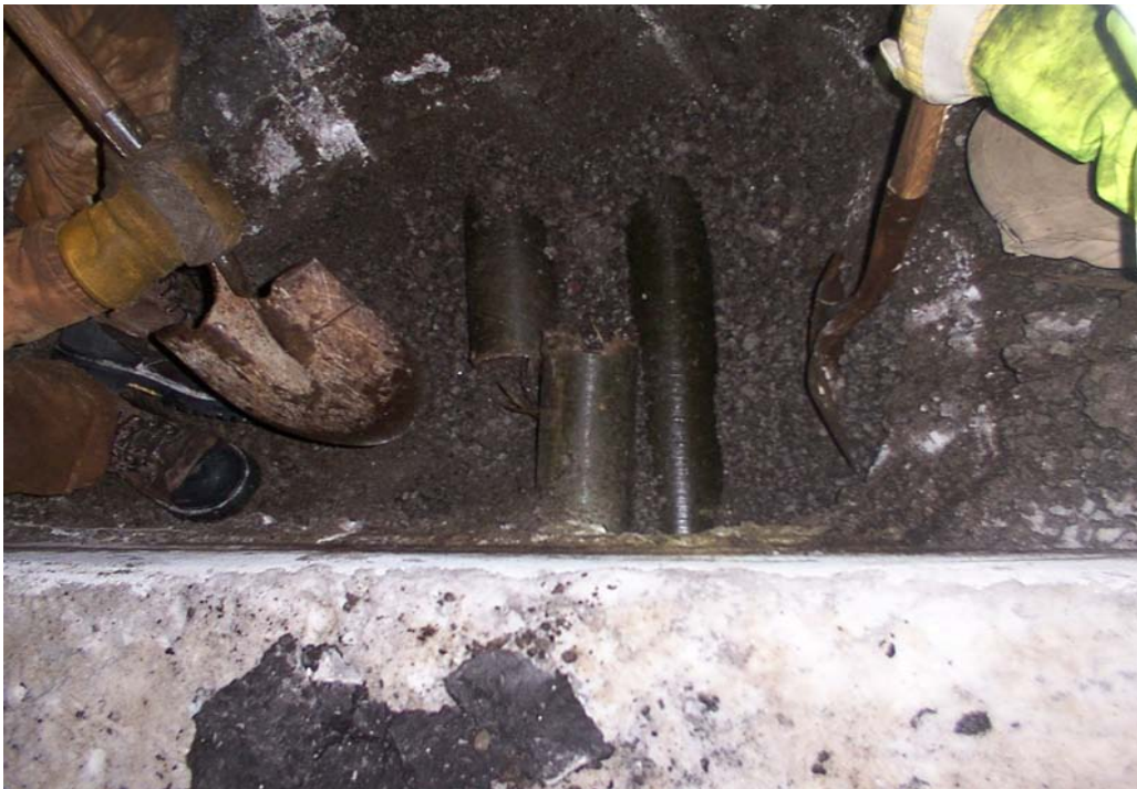
Photo 2 - View of furnace oil pipe break where 22,000L of furnace oil leaked into the subsurface.
