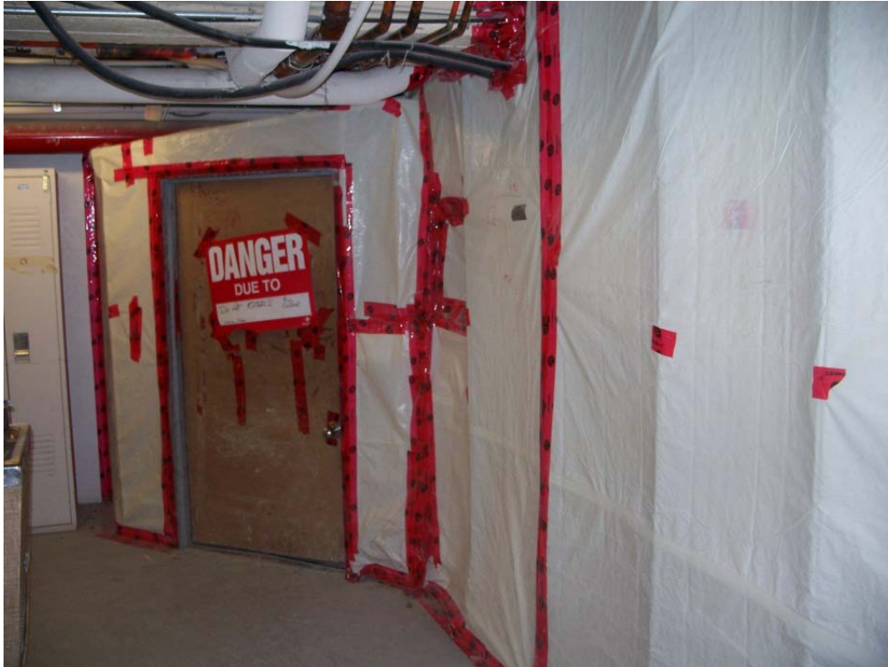
Photo 3 - View of elaborate infectious control system set up to permit the interior drilling of the 16 MPE recovery wells within the operating hospital.
